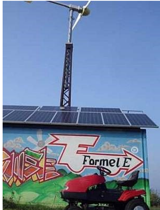
Windrad am Systemcontainer
